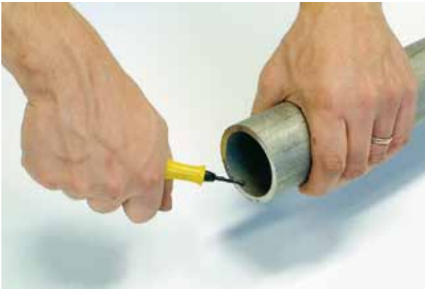
After cutting, the pipe is de-burred inside and outside; then wiped clean by cloth in order to remove any metal particles.
