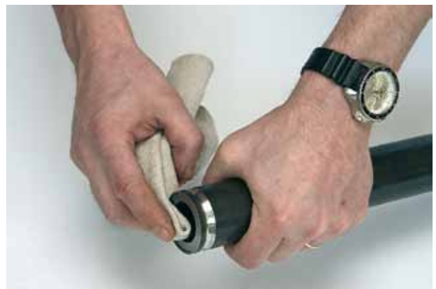
The cover is removed from pipe end and the pipe is cleaned with a doth.
